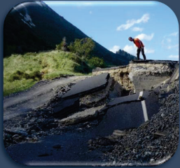
Seismic Surface Ruptures
